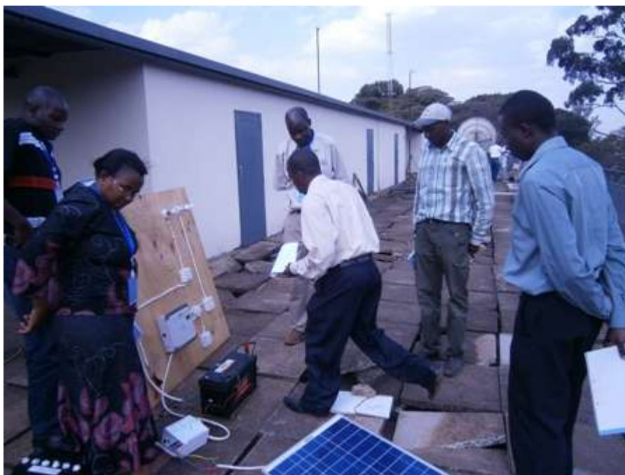
Figure 1 Some of the August 2014 solar academy participants installing a solar cell. For more photos see the August 2014 solar academy photo gallery .
