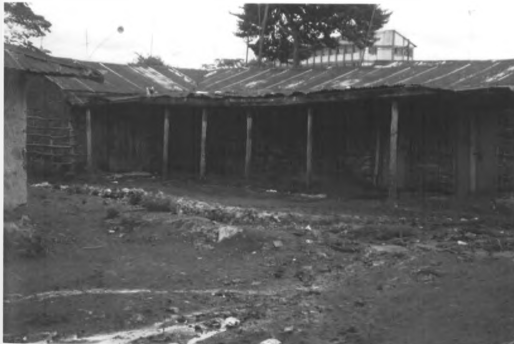
Figure 8: Poor quality of house walling materials
