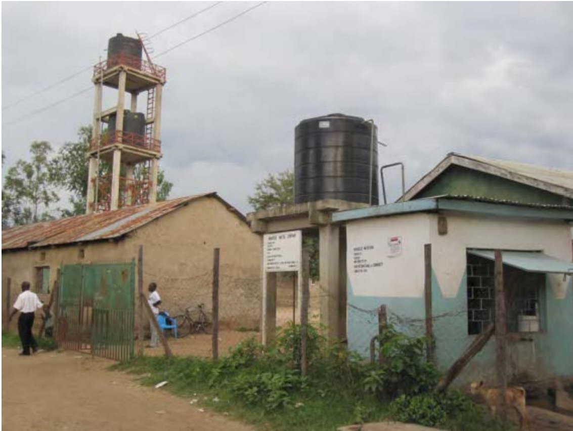
Photo 1 The Wandiege pumping station-cum-water kiosk (right) and the two 10,000 litres storage tanks [photo: Dick Foeken, 2012]
