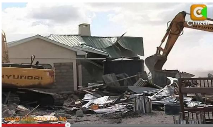
Plate 2: Result of Land tenure conflict - Syokimau case 2011
