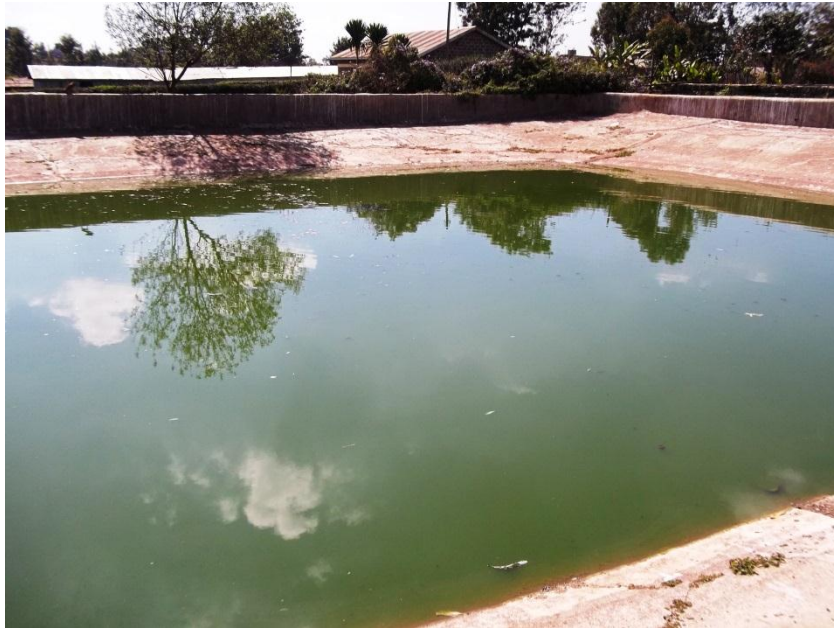
Plate 3: Maturation Pond at Dagoretti Slaughterhouse Wastewater Treatment Plant, Nairobi
