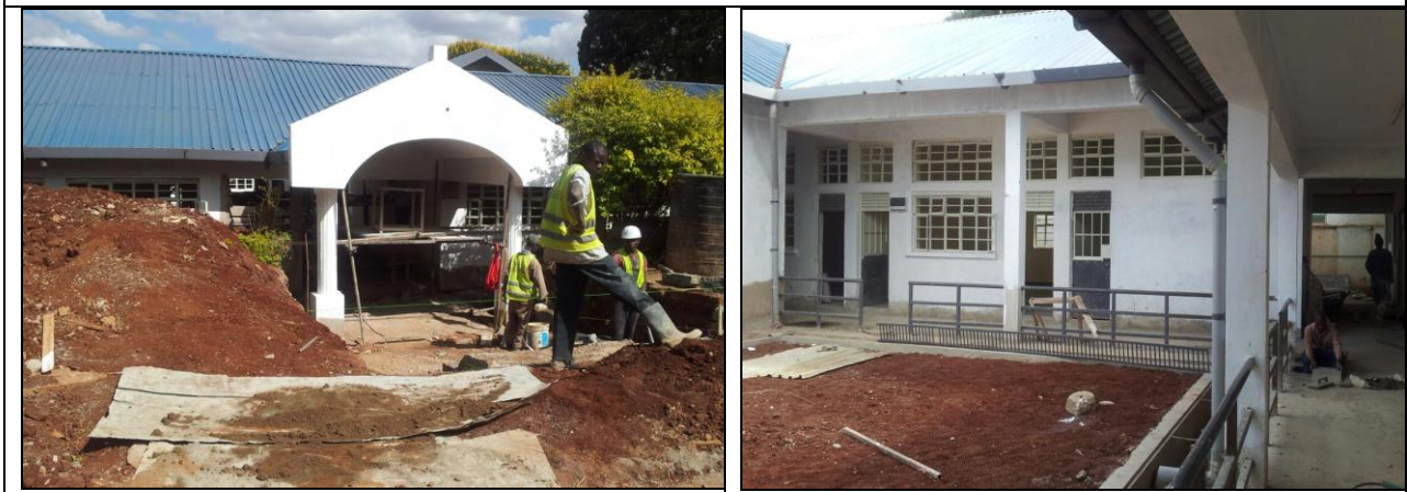
Phase II consisting of labs, offices and classes- Finishes and fitting works ongoing
