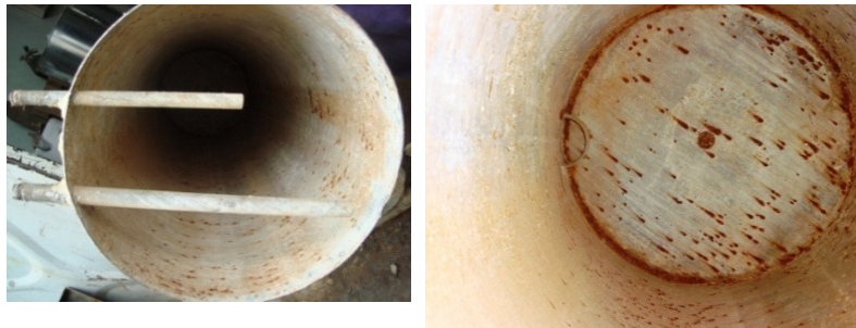
Figure 1.4: Images of a Corroded Tank (Courtesy: D&S 2012)
