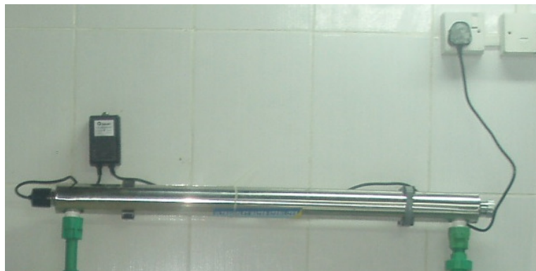
Figure 3.10: UV Chamber (Courtesy: Mag Utility Co. Ltd, 2014)
