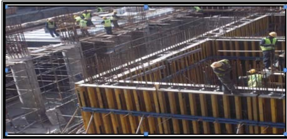
Plate 4.1: The 45 storey office building being put up in Upper Hill by Britam; Source: Field Data, 2014
