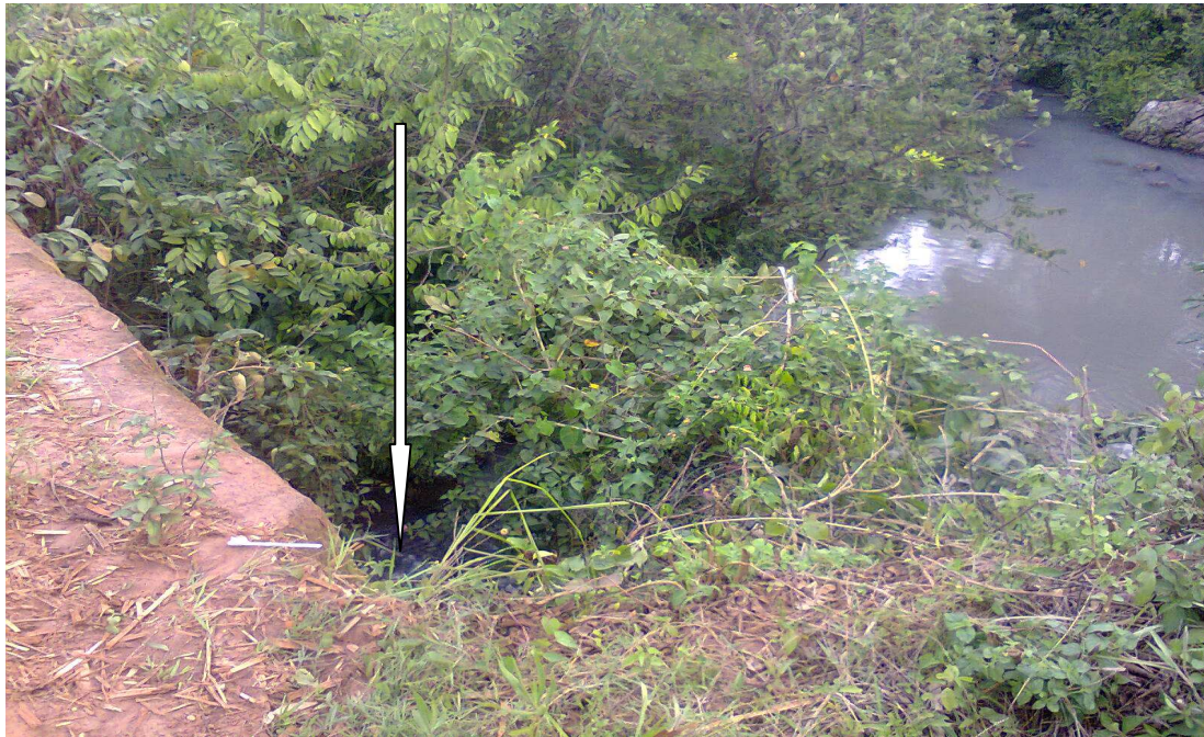
Figure 12: Picture of Kituni Bridge showing frequent accidental drowning spot
