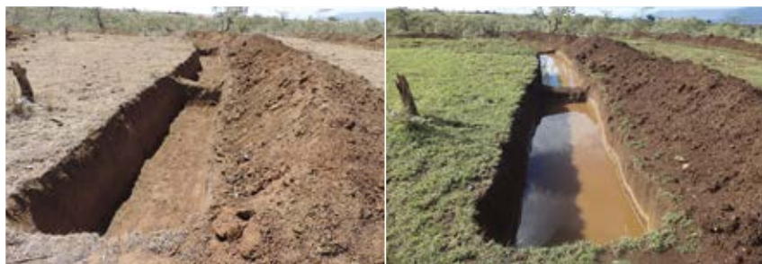
Plate 6 Established water retention ditches for rehabilitation of the Suswa gully in Narok.
