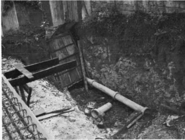
Private sewer connection on L.R. No. 2/61(Plot 176) Kirichwa Road
