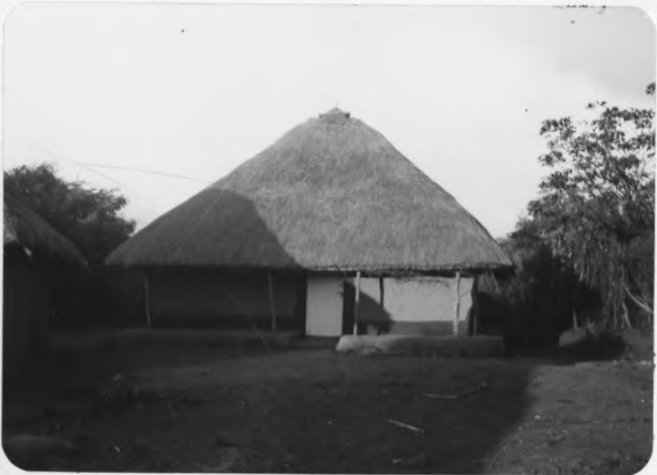
Plate 4: A house properly thatched and maintained. Although it is constructed using locally available building materials, it is of good quality.
