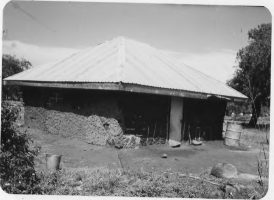
Plate 7: A house whose wall requires improvement in order to provide adequate shelter.
