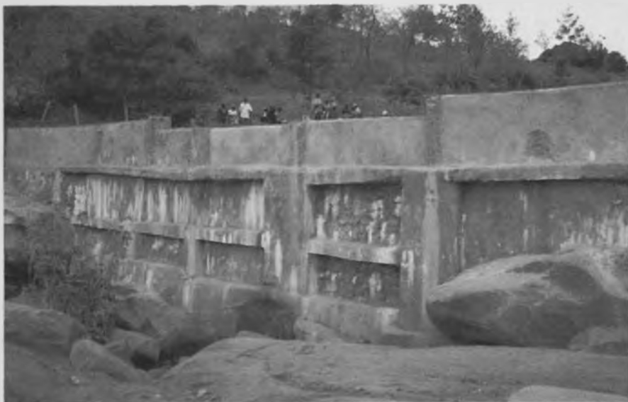
Photo 4.1: A check dam constructed by Meeko Ma Kwa Nduuka W.G at Kwa Nduuka along the Kaketa River
