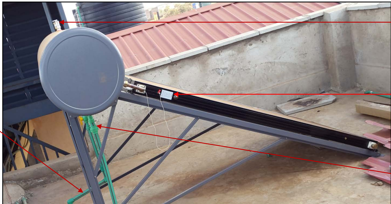
Fig.3.3. Flat plate collector SWH at the hotel
