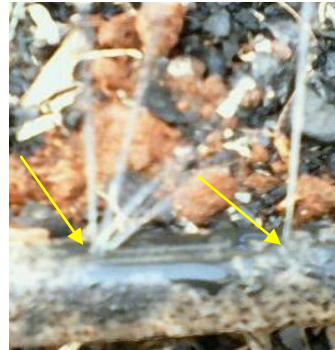
Fig.4.4 (b) Defective emitters
