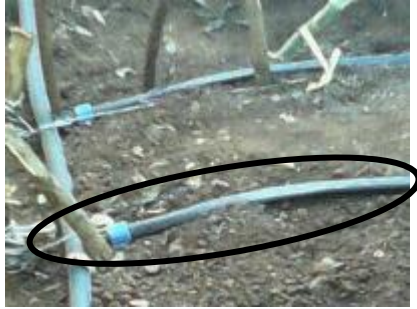
Fig. 4.4(e) Start connector not parallel to the bed restricts water flow
