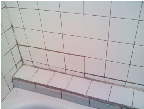
Figure 4.1: Uneven spacing between tiles
