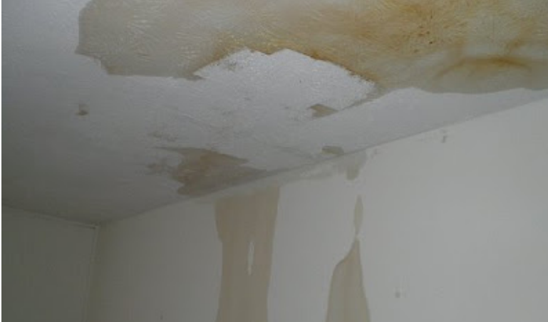
Figure 4.4: Leaks on ceilings and walls
