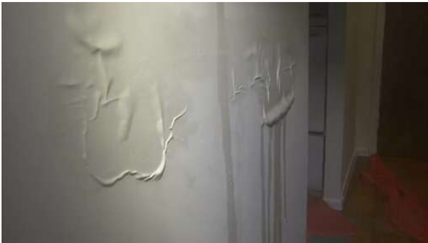
Figure 2.4: Peeling paint due to water leakage
