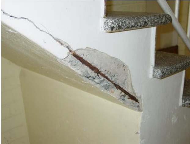
Figure 4.5: Exposed reinforcement bars
