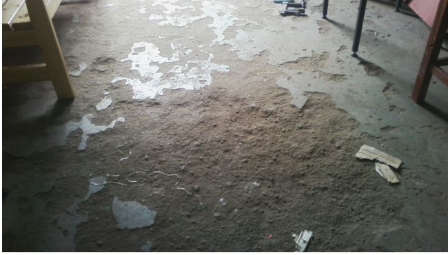
Figure 4.13: Loose floor screed and finish.
