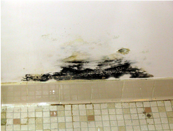
Figure 2.3: Black mold in wall
