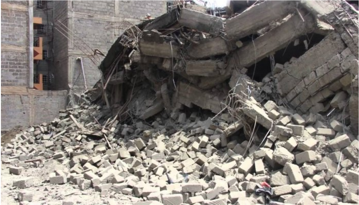
Figure 1.1 Collapsed Building in Nairobi
