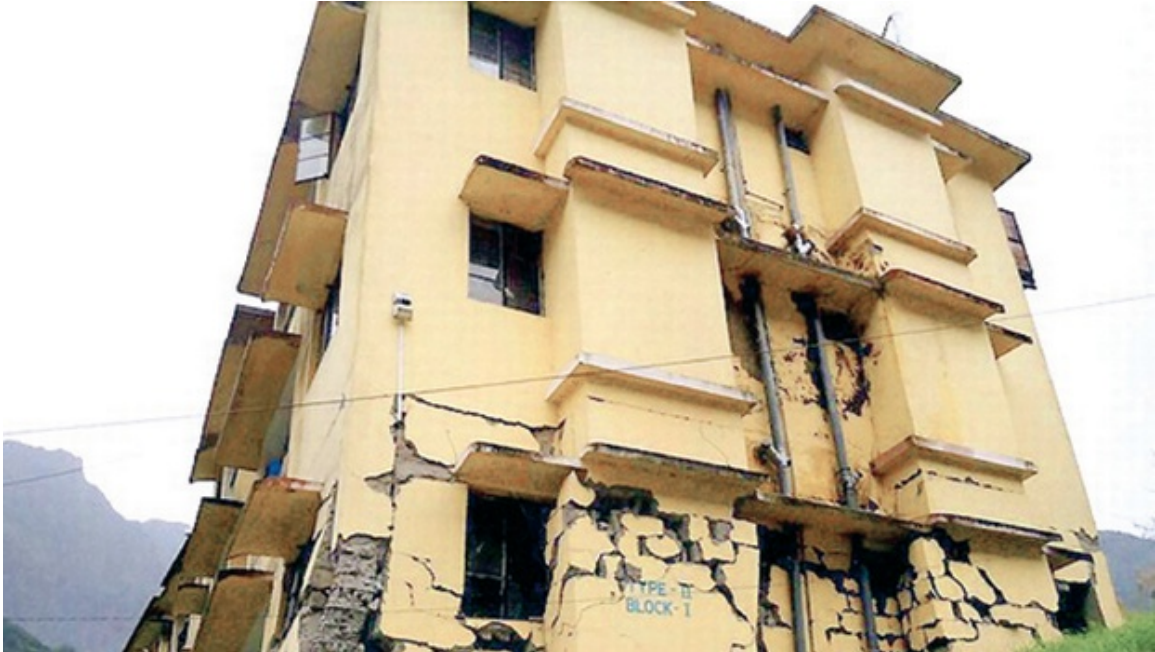
Figure 2.1: Cracks caused by faulty foundation
