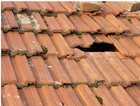
Figure 4.10: Poorly constructed and maintained roofs
