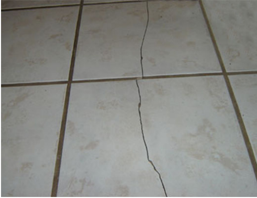
Figure 4.3: Cracks on tiles
