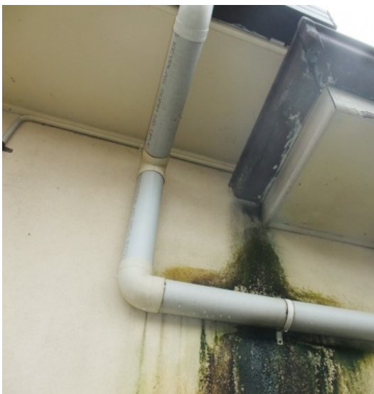
Figure 4.6: Leaking gutters & downpipes
