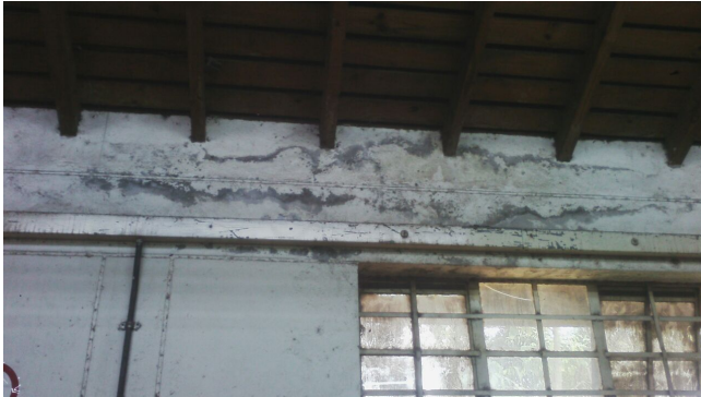
Figure 4.9: Leaking through walls
