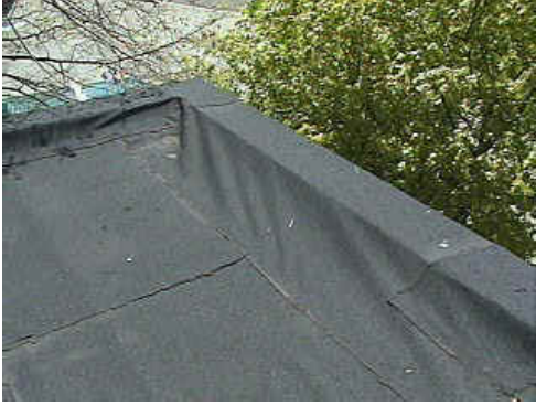
Figure 4.11: Poorly constructed roofs
